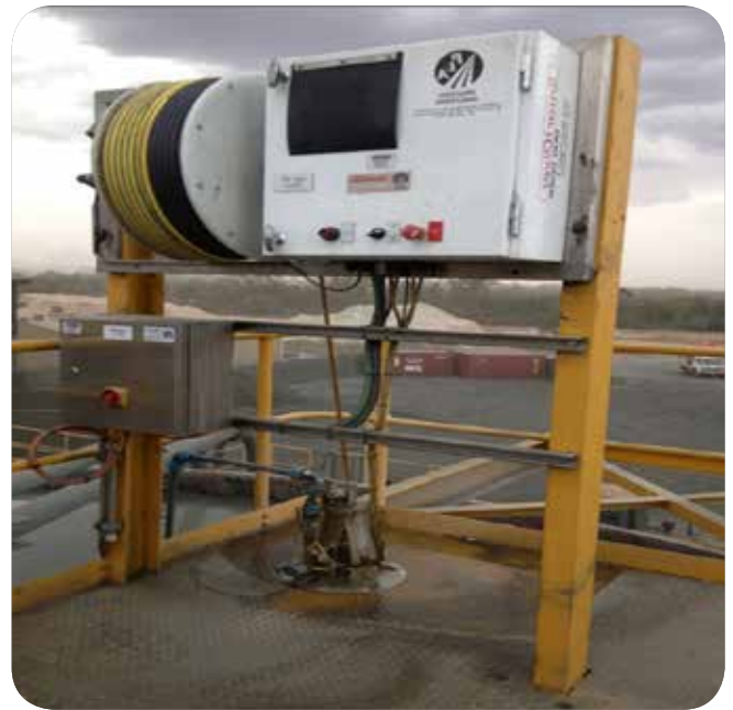
The Smart Diver as installed on-site at Peak Gold on the Tails Thickener
